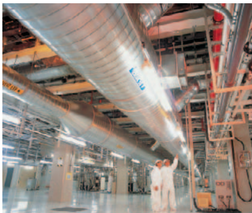
Stainless steel in a chemical installation
